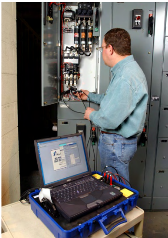
Technician is attaching current probes to de-energized power cables feeding a 75 horsepower motor
