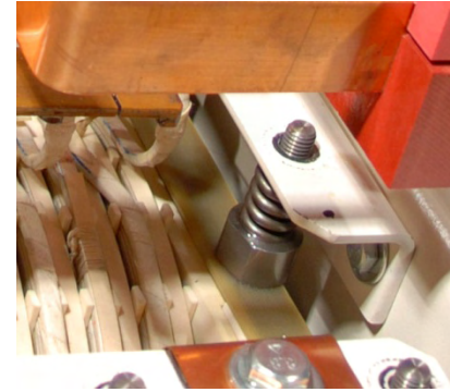
Fig 2: Fretted Bolts and Buckets
