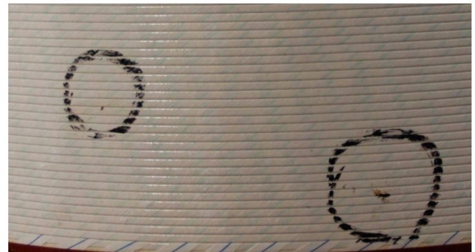
Fig 3: Burn Spots Between Primary Conductors
